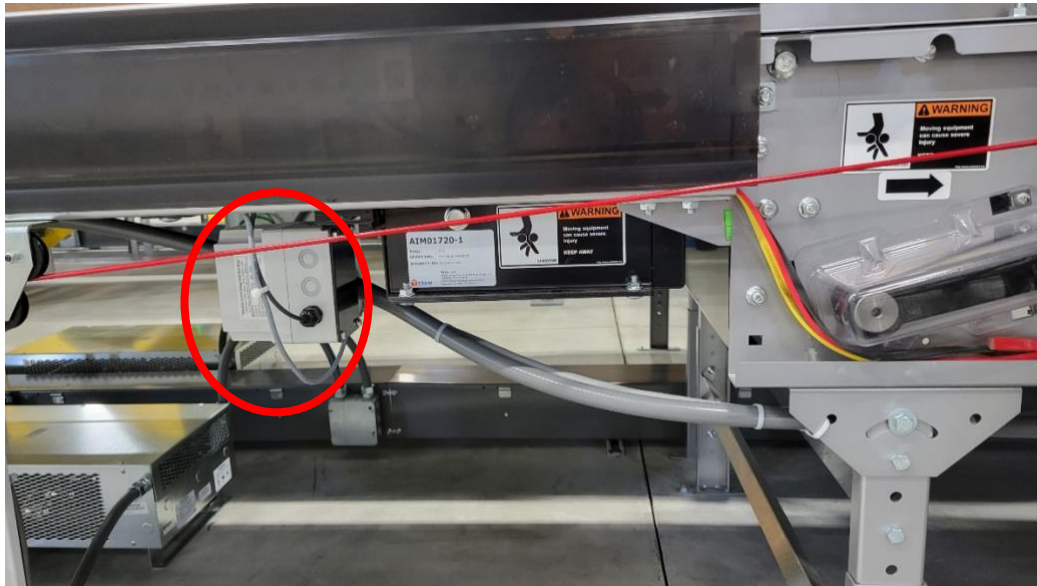
Figure 20: Installed AIMs Module
